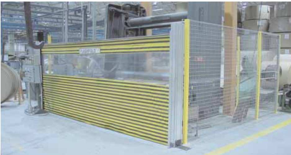
The Flash-Fold Barrier Door from Frommelt Safety Products remains closed when the paper slitter is in operation to prevent access to the machine. The remaining perimeter of the machine is guarded by the fixed Robo-Guard fencing to prevent unauthorized access.
